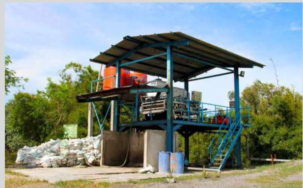
Belt presses are installed in some of our mills to help reduce effluent's COD load
