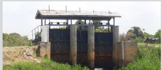
We install water gates to control the water level in our peat area
